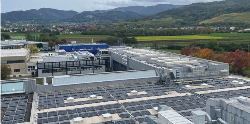
At our Freiburg, Germany, site, rooftop solar panels will generate renewable electricity to help power the facility.
